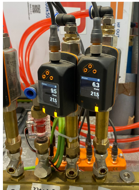
Figure 8. Pressure, flow, and temperature sensors.
